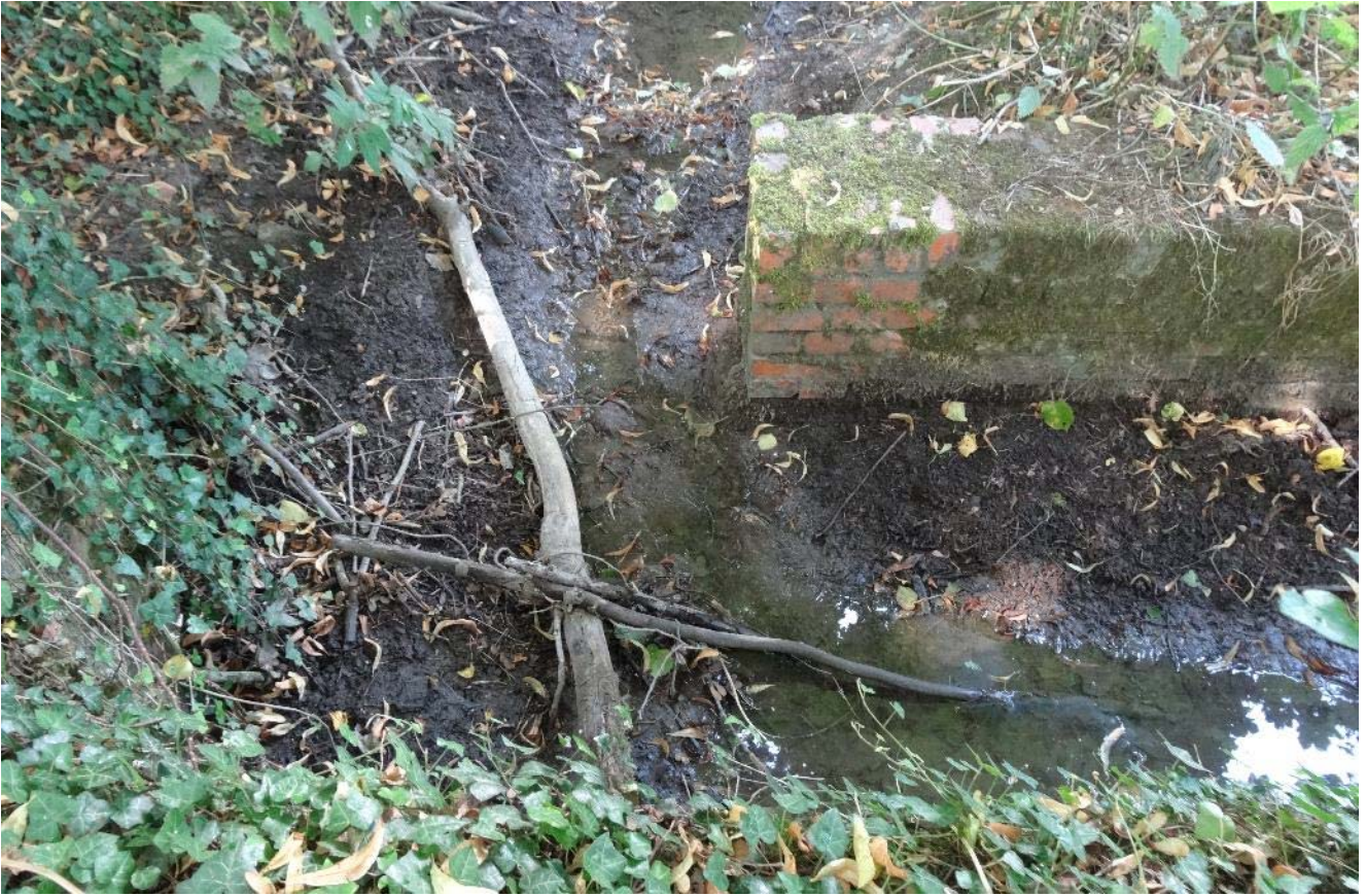
Photograph 8.6.10: Typical reach, with bank reinforcement evident along the left bank. Ryebridge Stream (facing upstream), 24/07/18, standard lens.
