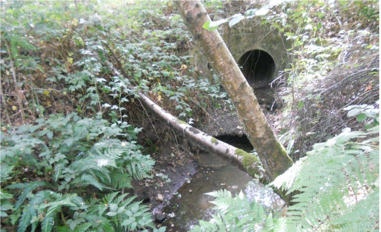
Photograph 8.6.15: The culvert beneath Aldershot Road, with undercutting of the downstream apron visible between the branch in the tree in the foreground. Gelvert Stream (facing upstream), 25/07/18, standard lens.
