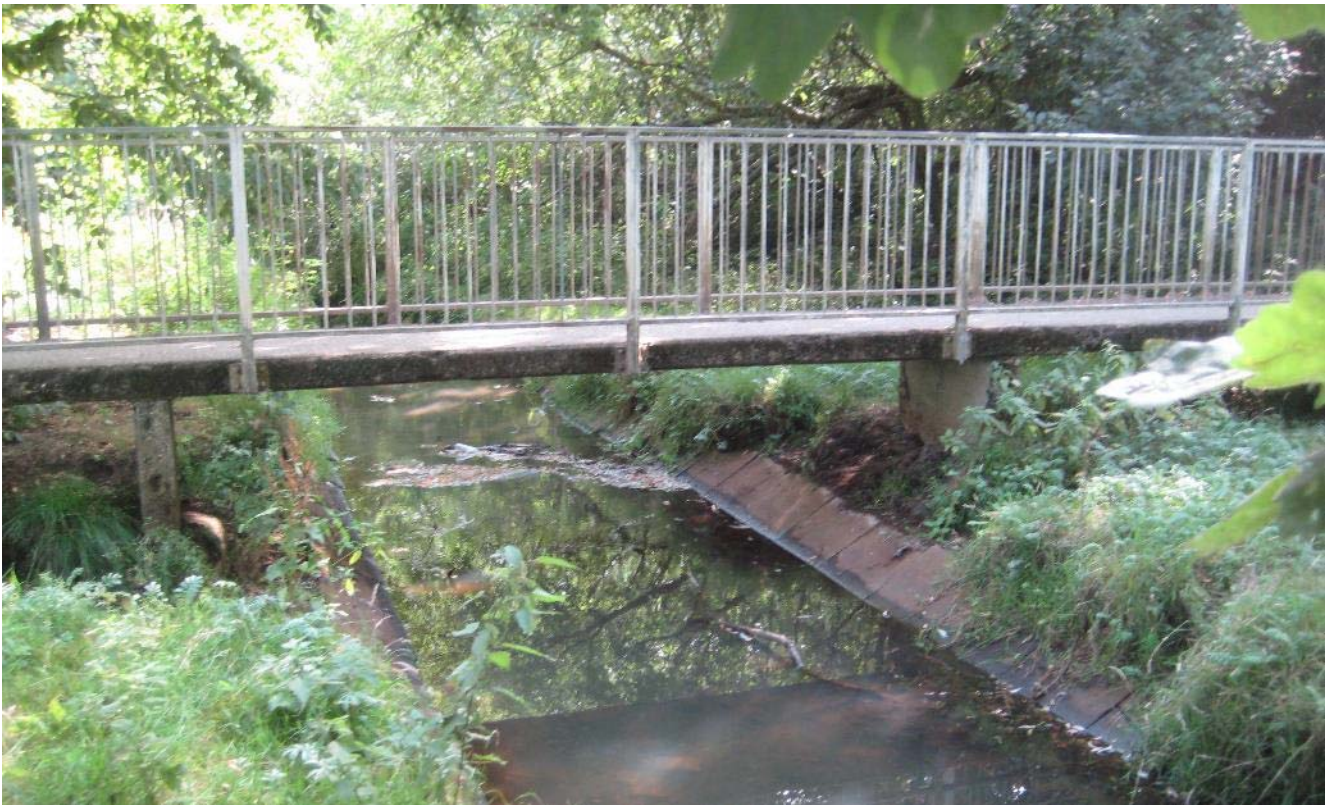
Photograph 8.6.18: Typical upstream reach, with footbridge and reinforcement evident along both banks. Cove Brook (facing downstream), 25/07/18, standard lens.
